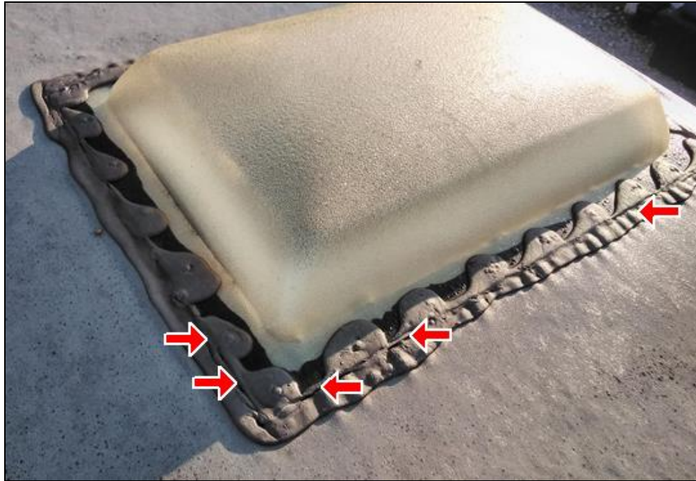
Rear of trailer Bathroom Skylight
