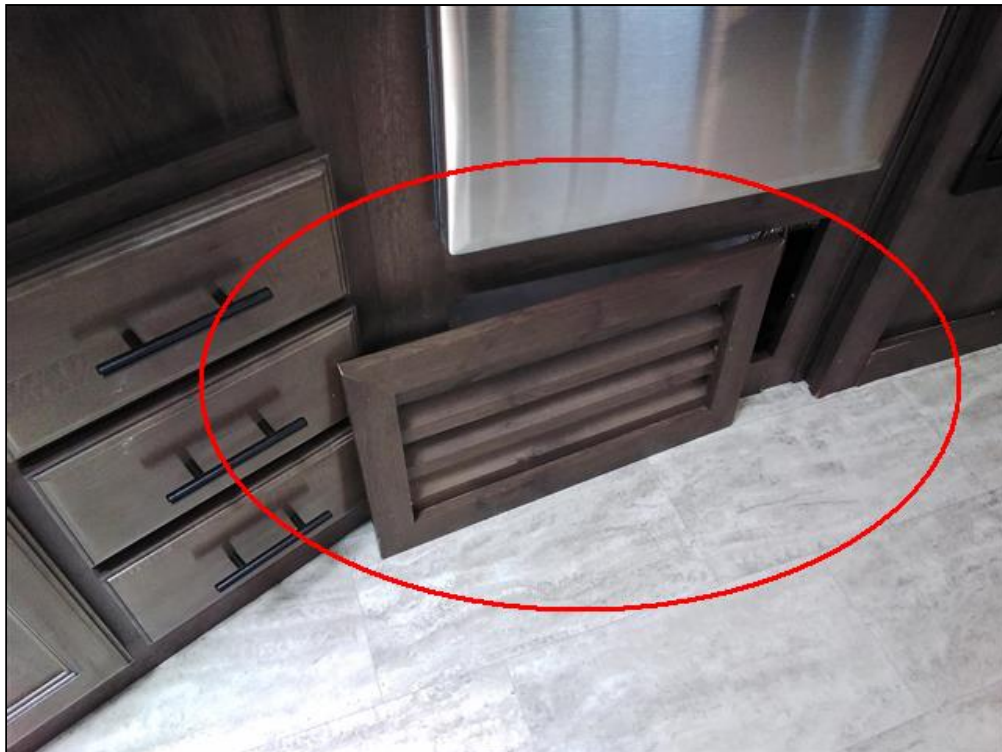
Furnace Air Intake Cover
