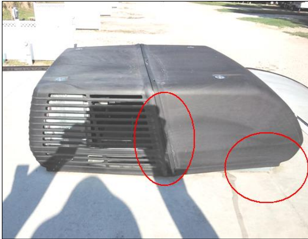
Front Air Conditioner
