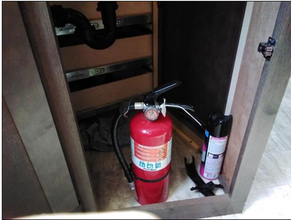
Fire extinguisher loose
