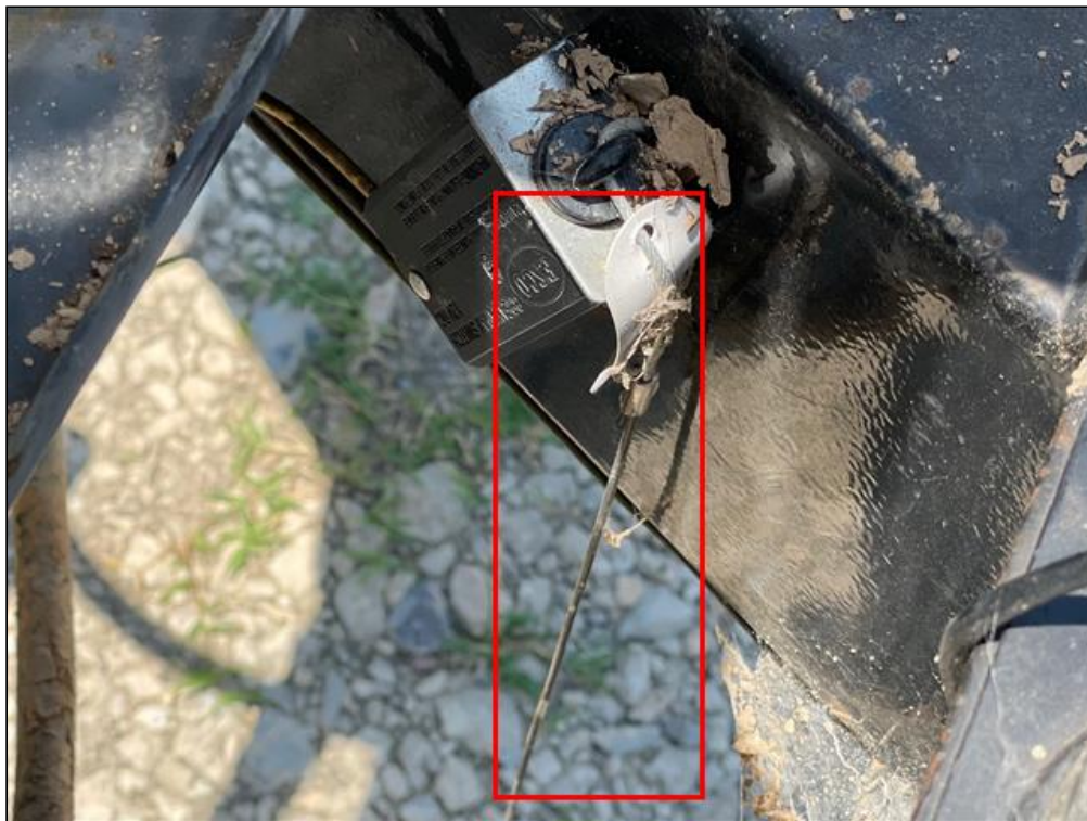
Cable in stressed position
