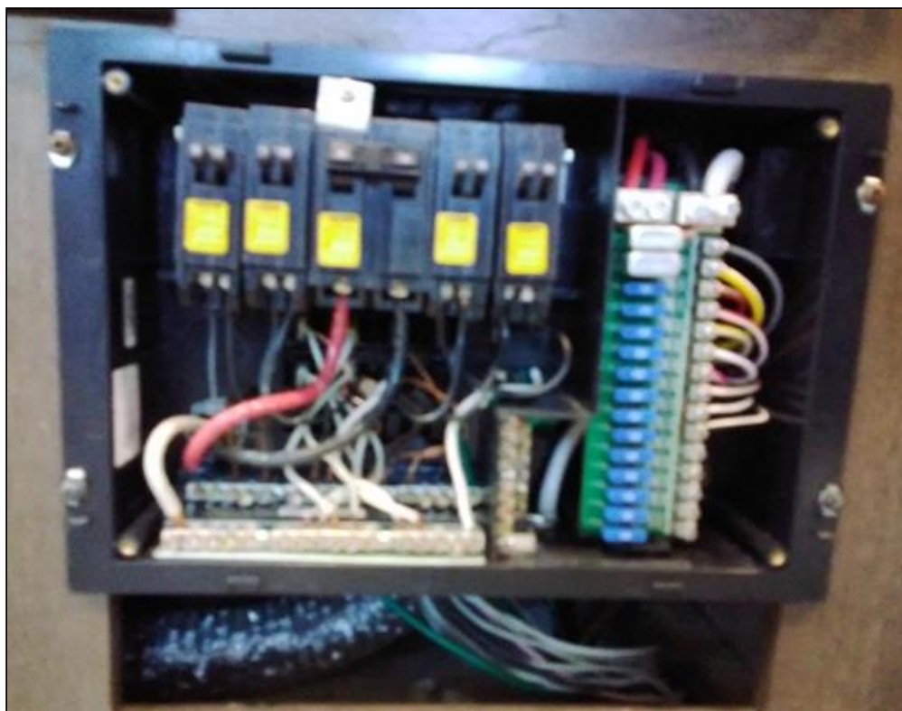
AC/DC Panel Box
